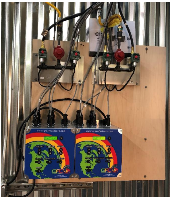
Picture 23: Control Panel and Gas Train Installation Example; follow all Local installation codes
